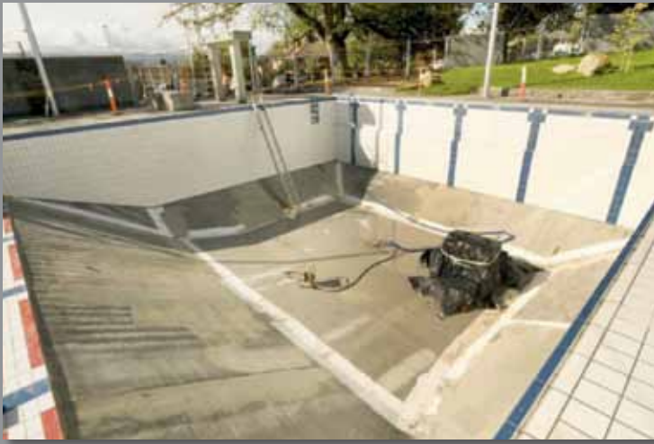
Leak sealing from the positive side – systems include injected expanding urethanes, epoxy injection, Crystal growth cementitious (Xypex)
