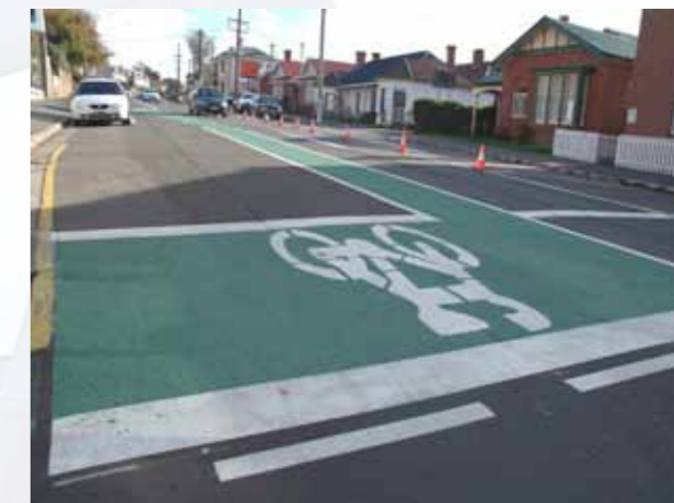
The cycle lanes along with adjacent centre line markings, including arrows & pedestrian markings, were all painted with TCP Degaroute long life cold applied plastic.
